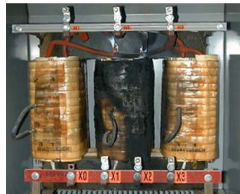
Fig. 1: View for defective transformer windings affected by short-circuits currents.
